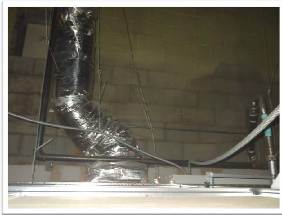
Photograph #005 View of above the drop type ceiling in the office and classroom renovation area.
