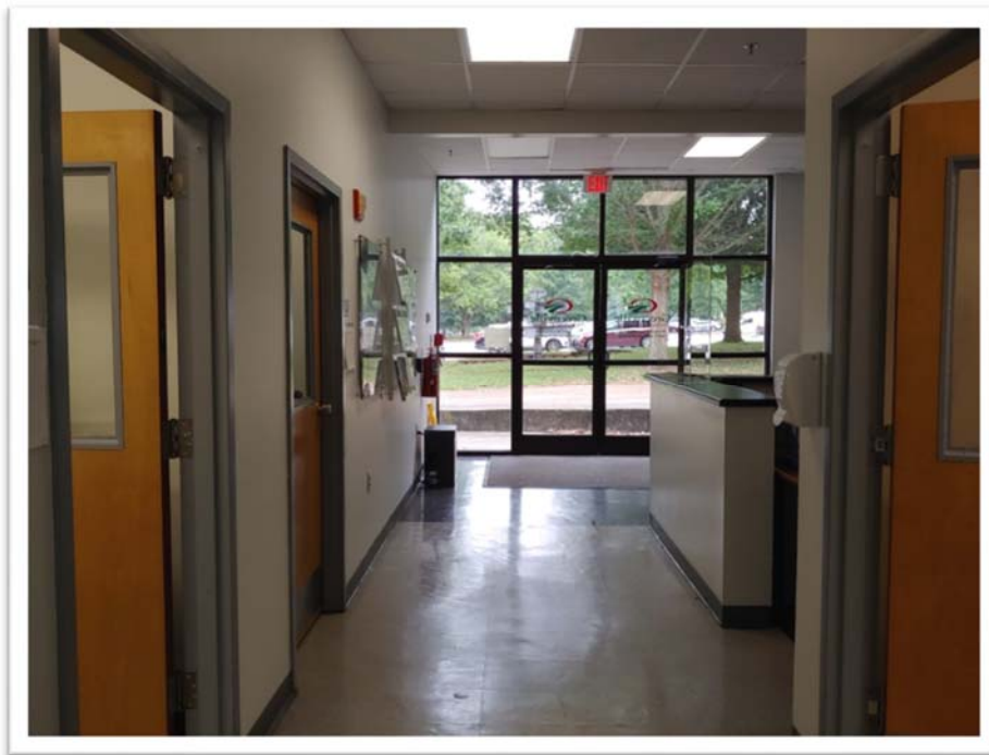
Photograph #002 View of the interior of the classroom and office area to be renovated in Area 5 on the northwest side of Engineering Technology Building 103.
